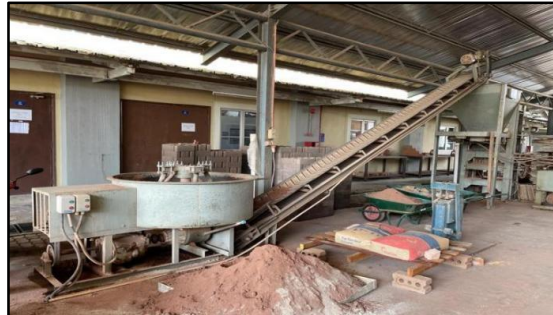
Figure 4: Conveyor and mixer machine
