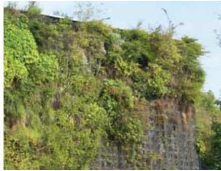
Figure 10: Damaged structure by living wall.
