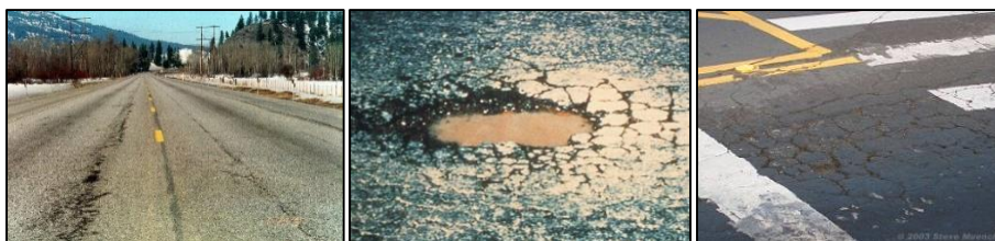
Figure 1: Pavement Distress Subjected to Moisture [11]
