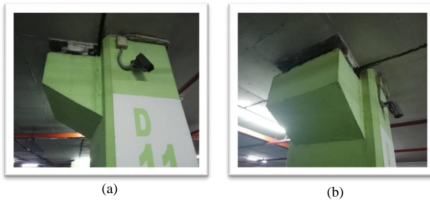
Figure 1: Single-sided reinforced concrete corbel at the basement carpark of Boulevard Shopping Mall, Kuching Sarawak.
