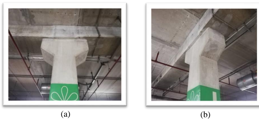
Figure 2: Double-sided reinforced concrete corbel at the basement carpark of The Spring Shopping Mall, Kuching Sarawak.
