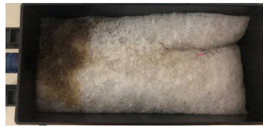
Figure 12: Filter Condition After System ON for Two days
