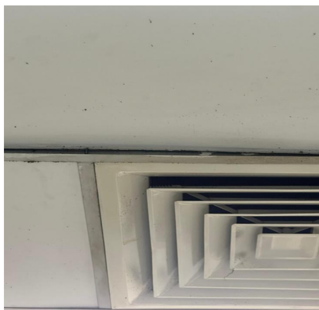
Fig 5 Dust buildup on the air-conditioning vent and ceiling surface
