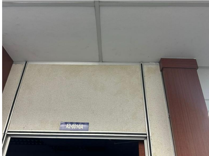
Fig 6 Dirty and slightly stained ceiling and wall area above the office door
