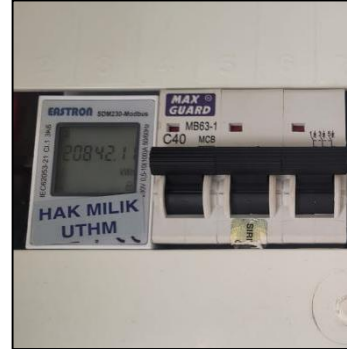
Fig. 8 Energy meter inside distribution box
