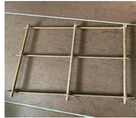
Figure 2: R6 steel bar has cut into suitable size and tie with the use of steel wire to produce reinforcement
