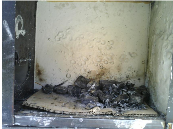
Figure 8: Combustion Chamber during the burning process
