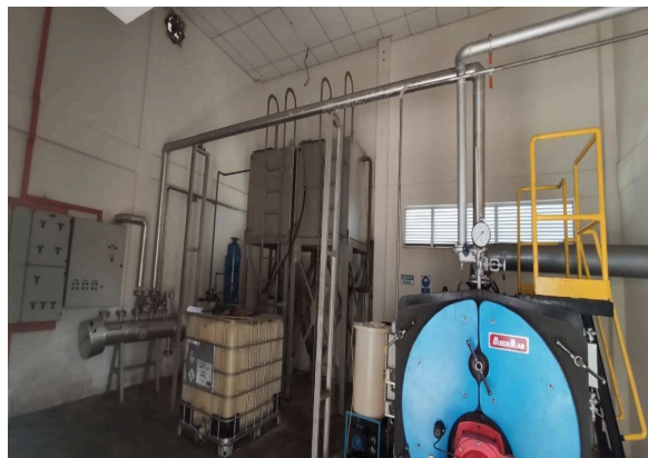
Figure 1: 2-inch A53 B carbon steel pipe outlet boiler to the steam header
