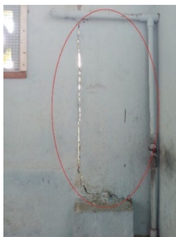
Figure 4: Combination of Vertical Crack and Diagonal Crack
