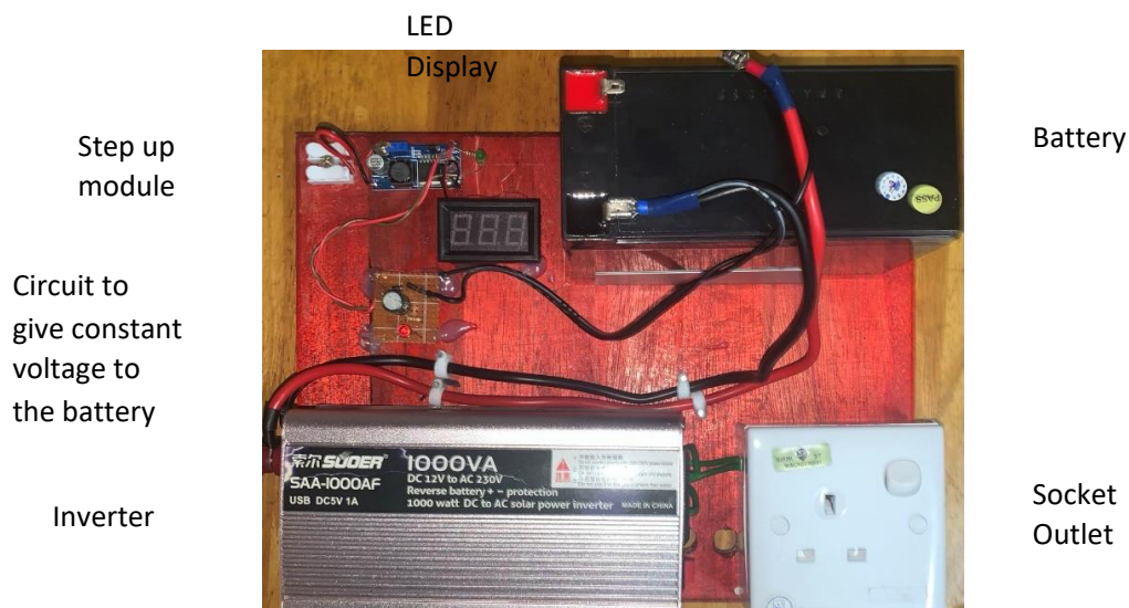
Figure 9: Complete set up of development of thermal energy harvesting from air conditioner for socket outlet application
