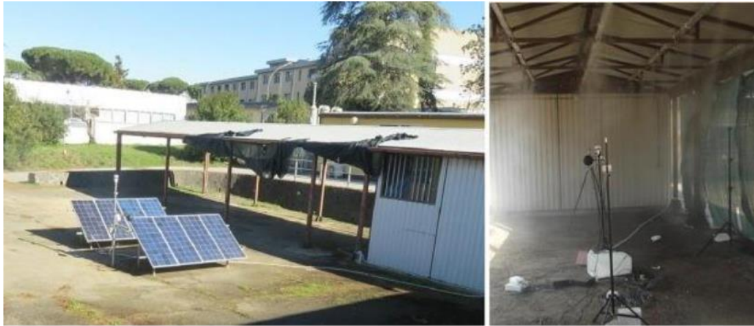
Fig. 2 Left photo shows the PV-powered misting system with battery storage, while the right photo shows the monitoring system in operation [15]
