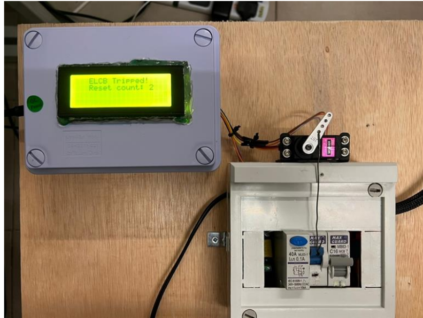
Figure 10: ELCB Tripped count 2
