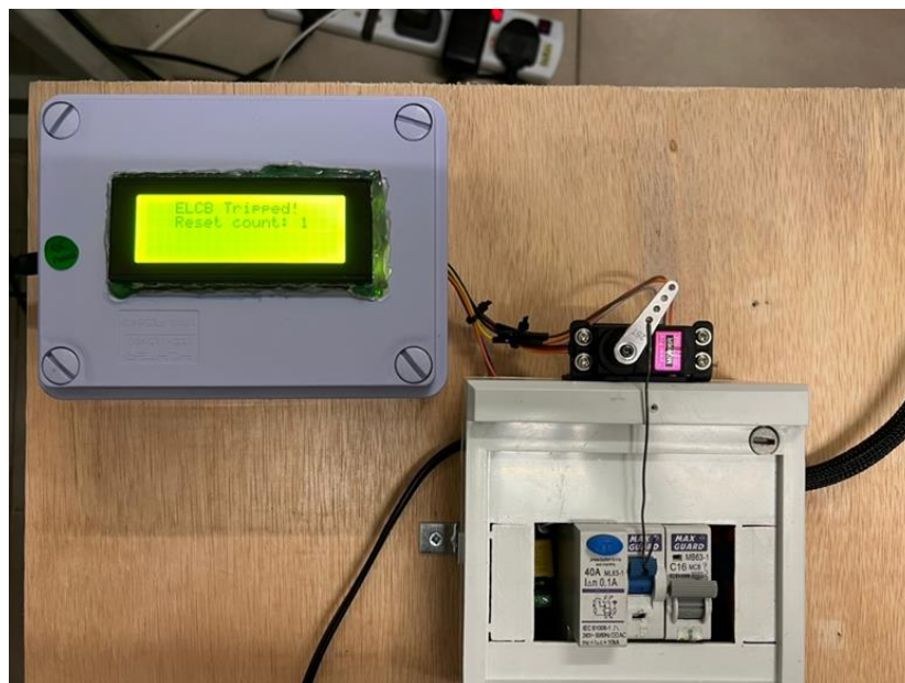
Figure 9: ELCB Tripped count 1
