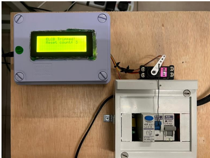
Figure 11: ELCB Tripped count 3
