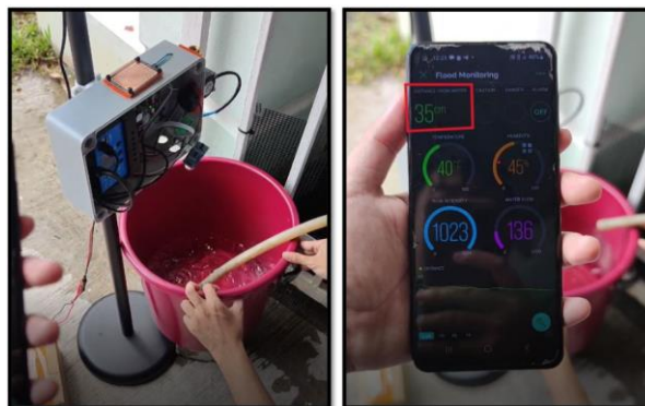
Fig. 10 Water level monitoring testing.
