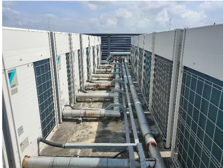
Fig. 16 VRF system used by office building
