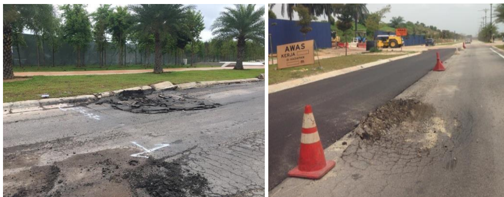
Fig. 1 - Pavement failure at Panchor-Muar road
