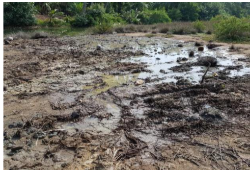
Fig. 2 - Inland side of SCE that occur seepage [4]
