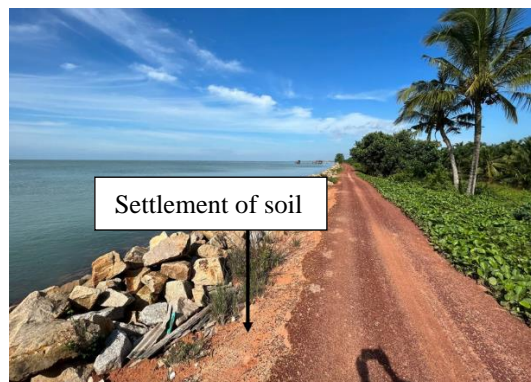
Fig. 3 - Seaward slope of SCE that occur settlement
