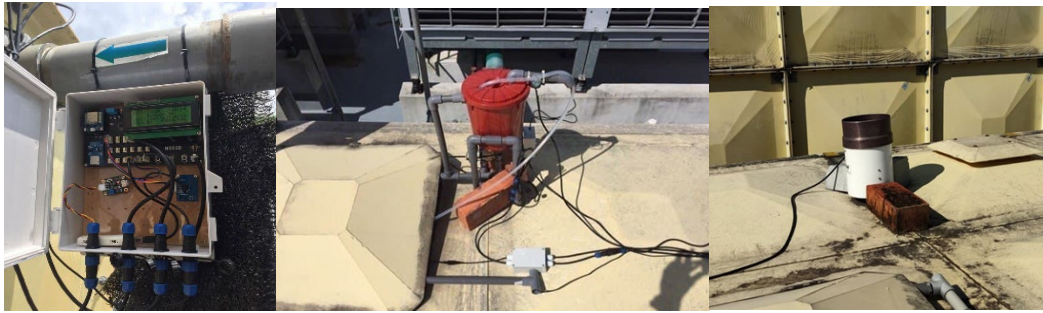
Fig. 4 - Location of IoT system installed at the RWH storage tank
