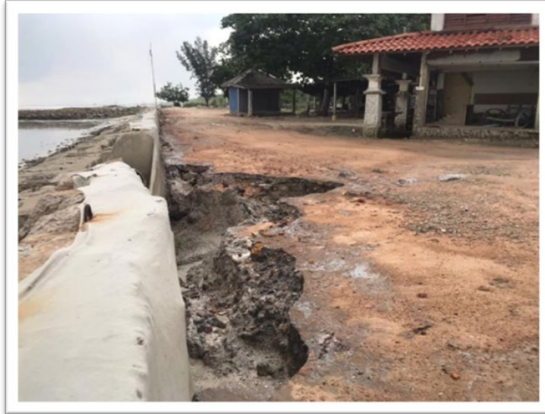
Fig. 1 - Pantai Punggur shoreline erosion in April 2021
