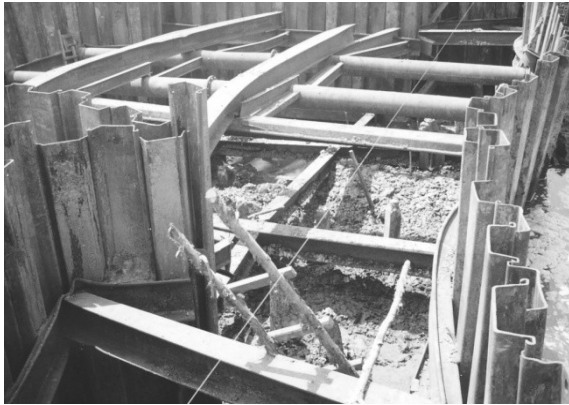
Fig. 13 Failures of sheet piles in soft soils due to deep sliding underneath the structure in Surabaya (photographic documentation, Rahardjo).
