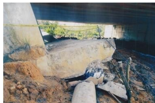
Fig. 24 Lateral displacement of bridge foundation [21]
