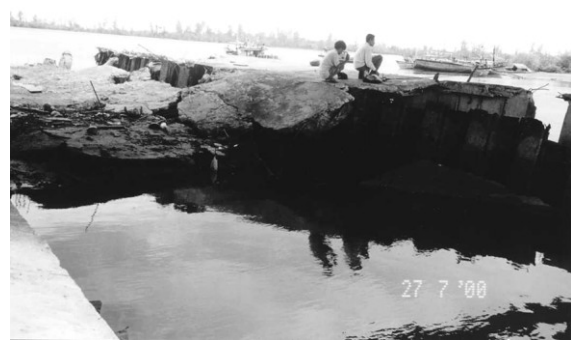
Fig. 31 Failures of sheet piles due to liquefaction (photographic documentation, Rahardjo)
