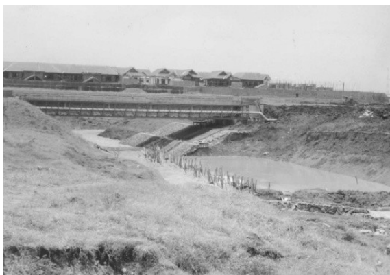
Fig. 14 Failures of abutment fill due to soil softening (photographic documentation, Rahardjo).
