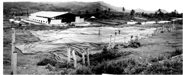
Fig. 18 Emergency action for handling landslide in Purwakarta by Temporary Cover [14].
