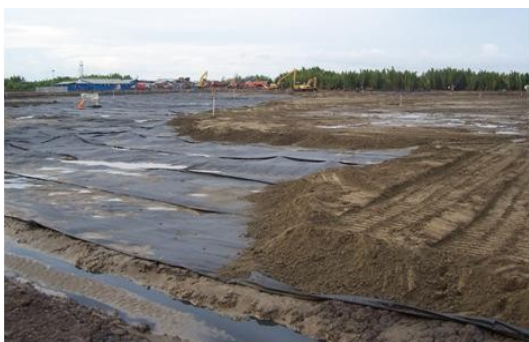
Fig. 10 The use of geotextile for separation between foundation soils and the backfill material
