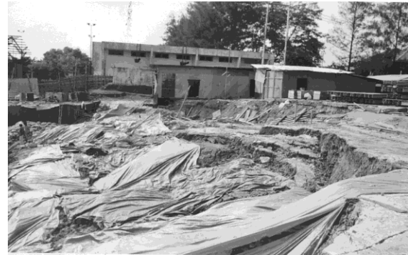
Fig. 11 Slope failures during excavation for basement in Surabaya (photographic documentation, Rahardjo)
