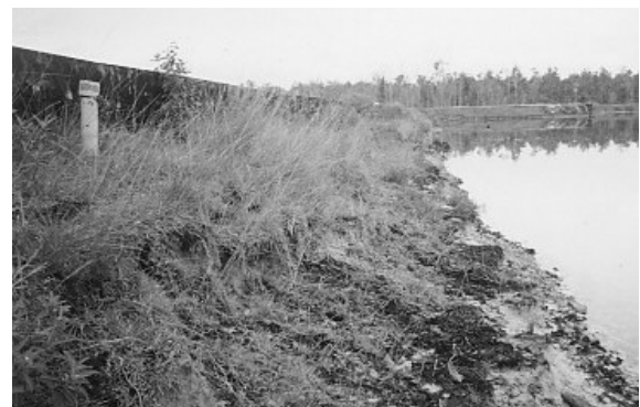
Fig. 15 Embankment failures due to soil dispersions at Samboja Dam, East Kalimantan (photographic documentation, Rahardjo).
