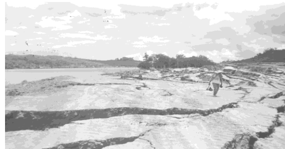
Fig. 8 Failures of fill constructed on soft soil foundation in Mahakam River, East Kalimantan (photographic documentation, Rahardjo).
