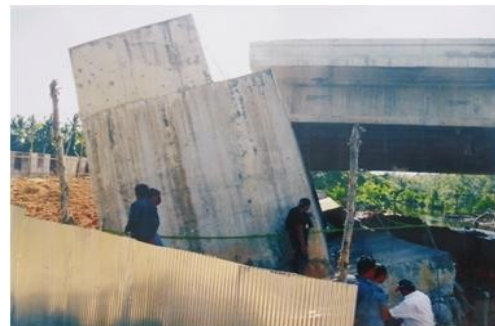
Fig. 23 Failures of bridge abutment [21]
