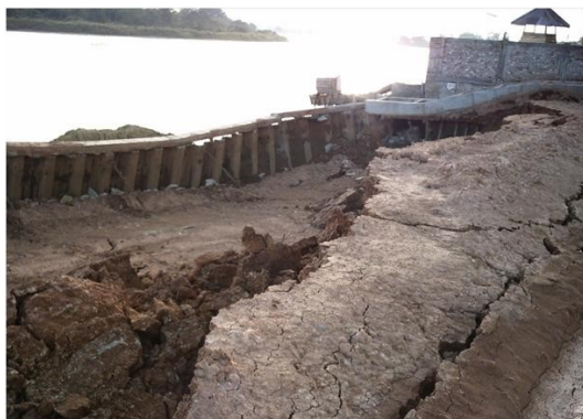
Fig. 26 Failures of sheet piles due to excess pore pressure during fill placement.
