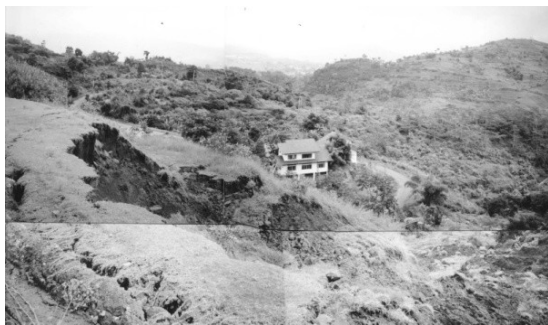
Fig. 21 Sliding of poorly compacted fill material in Cipanas, West Java (photographic documentation, Rahardjo).
