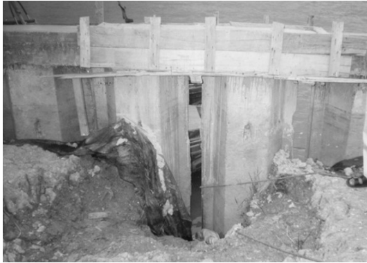
Fig. 25 Failures of sheet piles due to excess pore pressures during fill placement in Palembang (photographic documentation, Rahardjo).
