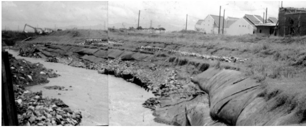
Fig. 32 Failures of earth reinforced embankments (photographic documentation, Rahardjo).
