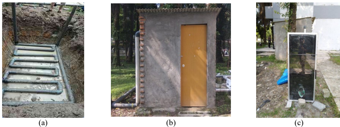
Fig. 1 - (a) EAHE pipe; (b) testing room; (c) solar collector
