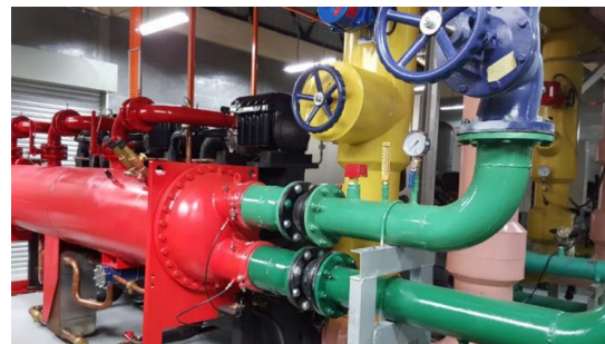
Fig. 8 - Hospital Teluk Intan applying Centrifugal Chiller with Magnetic Bearing
