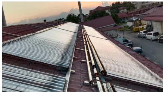
Fig. 7 - Solar Collector for hot water system at Hospital Sarikei Sarawak
