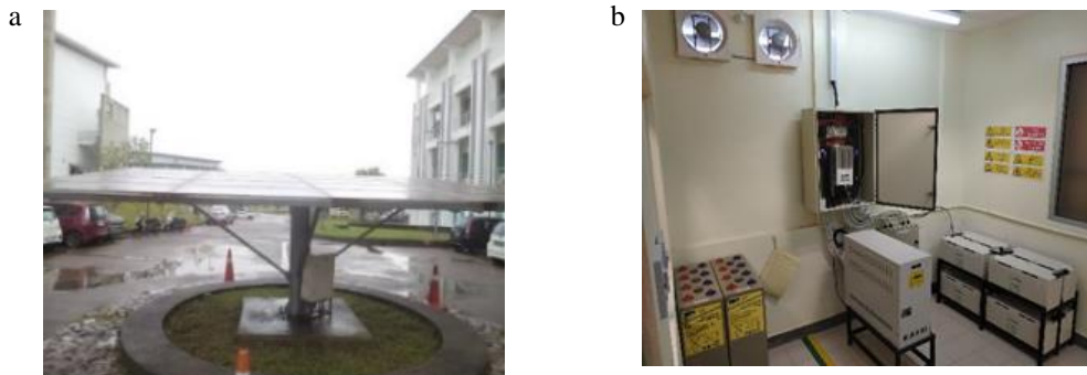
Fig. 7 - (a) Combined Solar Panel; (b) System Controlling Room
