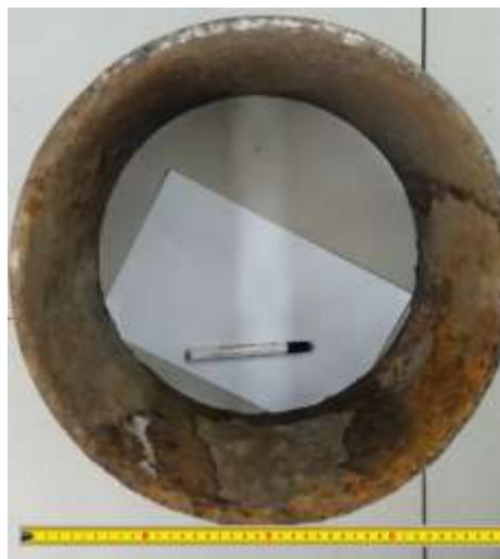
Fig. 2 - A sample cut of the pipe from the condensate pipeline
