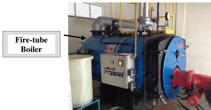
Fig. 1 – Fire-tube boiler located in UTHM Biodiesel Plant
