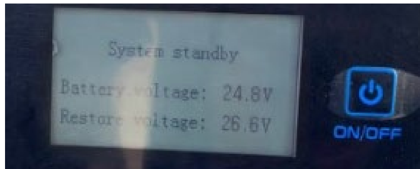
Fig. 4 Results of battery voltage and restore voltage from solar PV system
