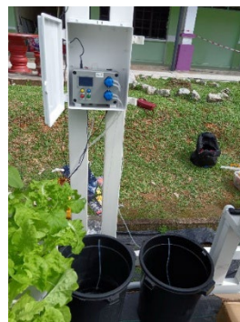
(b) Automatic mixing system
