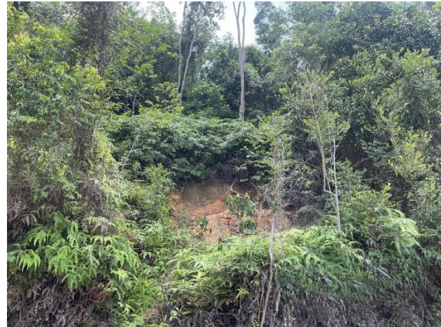
Fig. 4 Slope failure along the survey line
