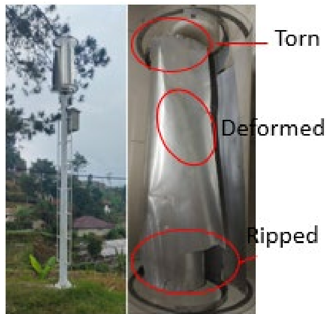
Fig. 3 The damage of turbine blades due to wind speeds far exceeding normal wind speed limits [14]
