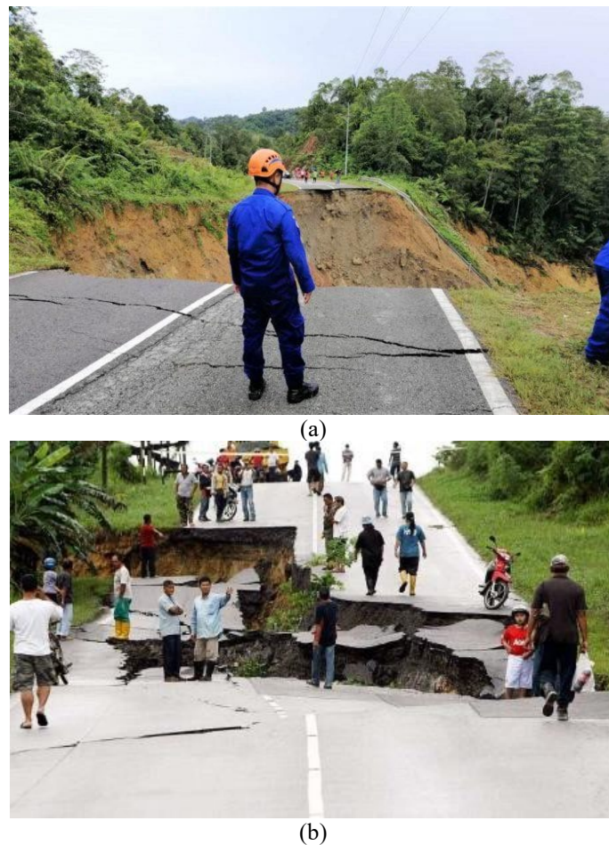
Fig. 1 - Example of slope failure reported along Sarawak roads in year (a) 2020 [16], and; (b) 2011 [17]
