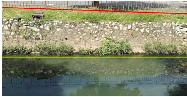
Fig. 4 - Riverbank Edge (Red line) and Waterline Edge (Yellow Line) from outdoor location of the IoT edge computing
