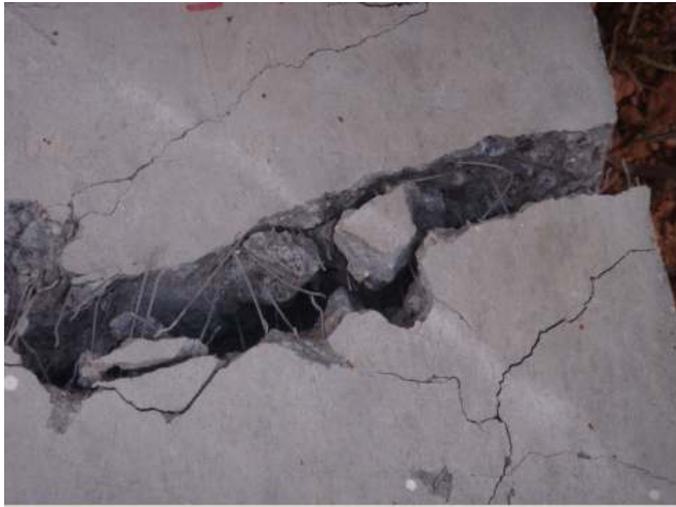
Figure 12: Fiber pullout from the concrete due to explosive loading.
