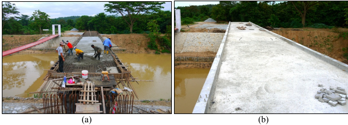
Figure 9: (a) Concreting of first half of the deck, (b) RC deck completed.
