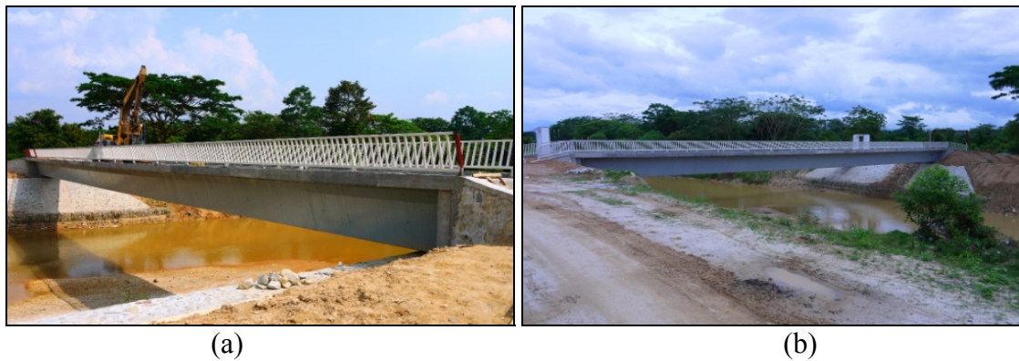
Figure 11: (a) One 22 tonnes excavator place at the bridge midspan and (b) completed bridge open for traffic.
