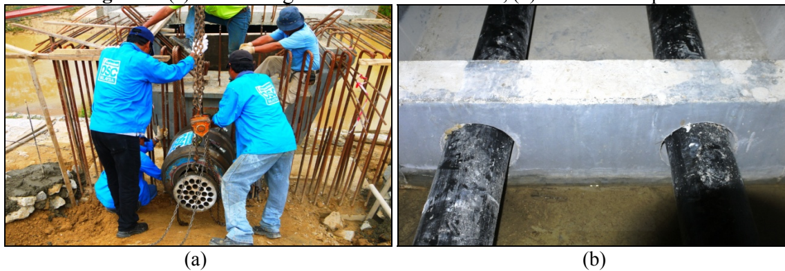
Figure 10: (a) Stressing technician preparing for second stage post-tensioning and (b) no sign of major cracking at the deviator.
