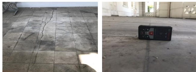
Fig 2 - Structural crack, slanting of floor slab, and fallen ceiling detected during the walk-in survey
