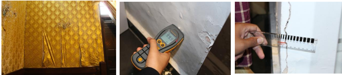
Fig 6 - Defects that were detected during the walk-in survey (dampness) and could be tested using a non-destructive test
