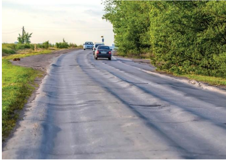
Fig. 1 - Rutting problem on the asphalt surface (Daniel, 2017)
