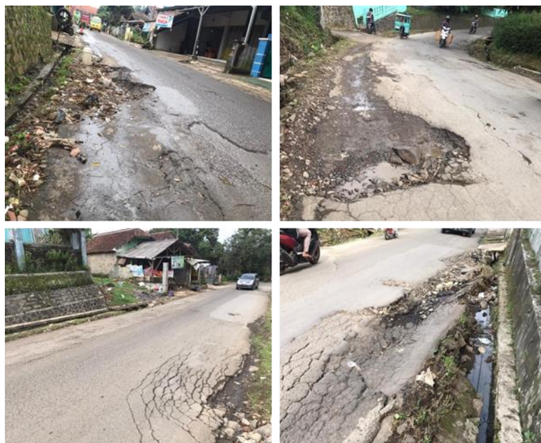
Fig. 2 - Pavement distresses in Cikalong-Cipeundeuy road
