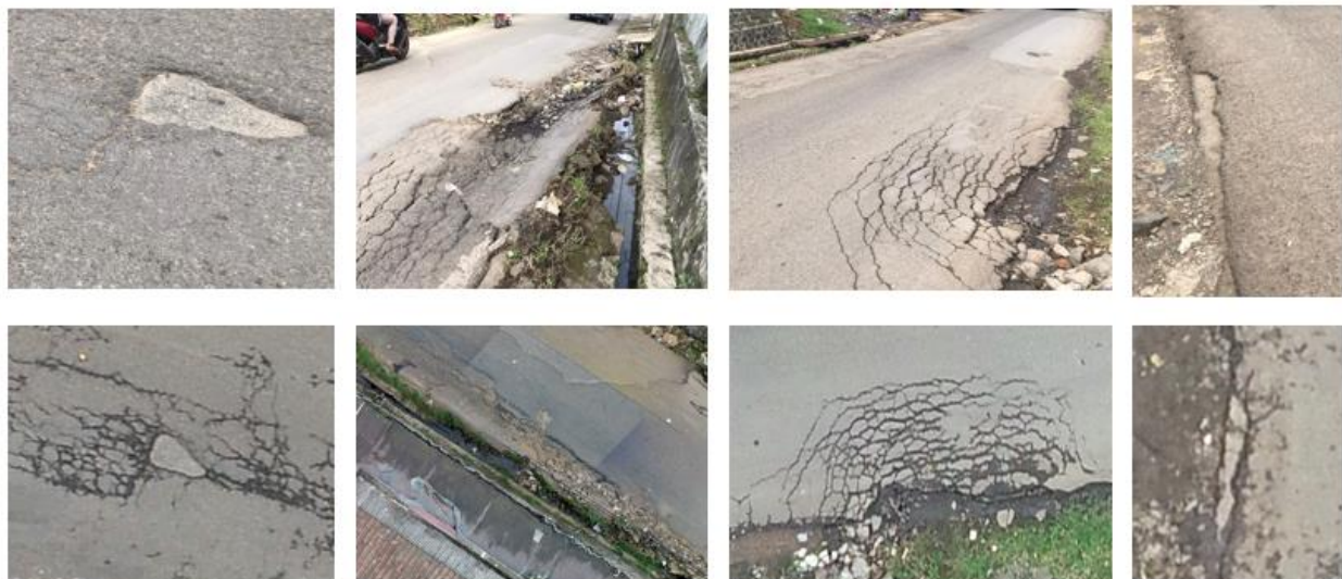
Fig. 5 - The results of the identification of the types of pavement distress in the 3D model (below) to the real conditions in the field (top). Left – Right: pothole, depression, edge cracking
