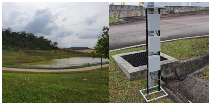
Fig. 3 - Real System with sensory network at Field implementation Water Retention in UiTM Pasir Gudang
