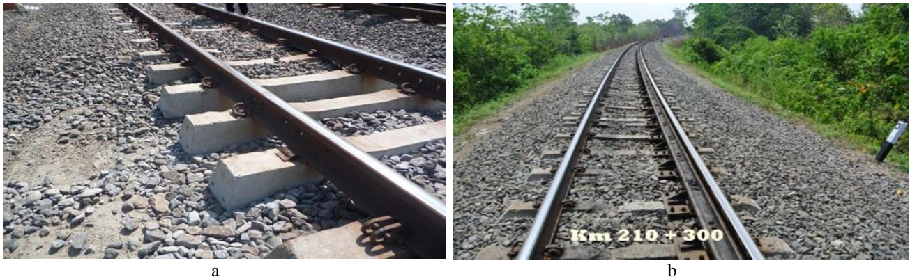
Fig. 1 - Some examples of black spots in Indonesia’s conventional track line: (a) lack of ballast materials; (b) broken concrete sleepers after train derailments
