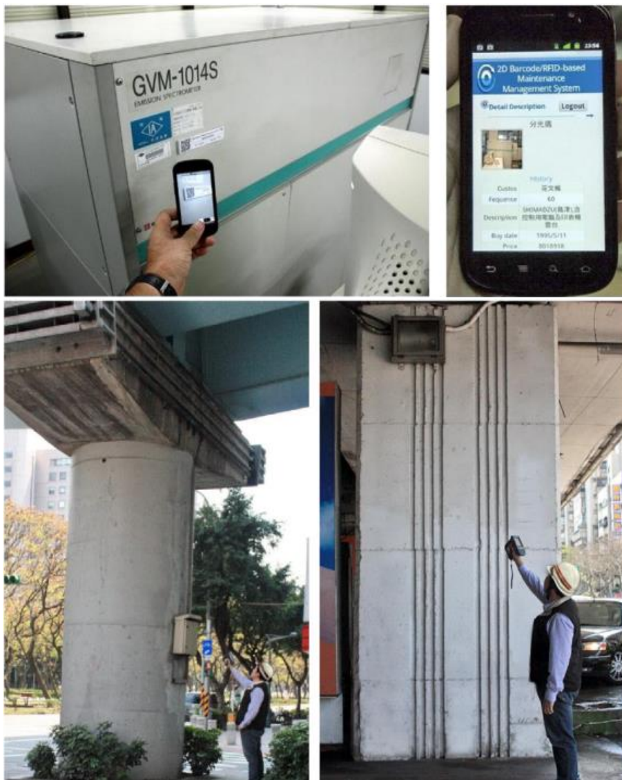
Fig. 3 - Applying Barcode (Barcode), Radio frequency identification (RFID) technologies to identify equip-
